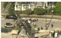
VIDEO/ Crane collapses onto a car in Miami, operator jumps from cabi...
